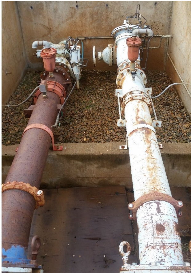
Figure 2-2 – Raw Water Intake Pump Station
